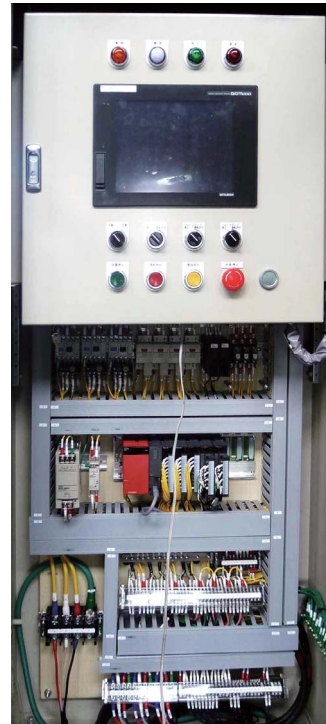
Control devices (Control panel)
